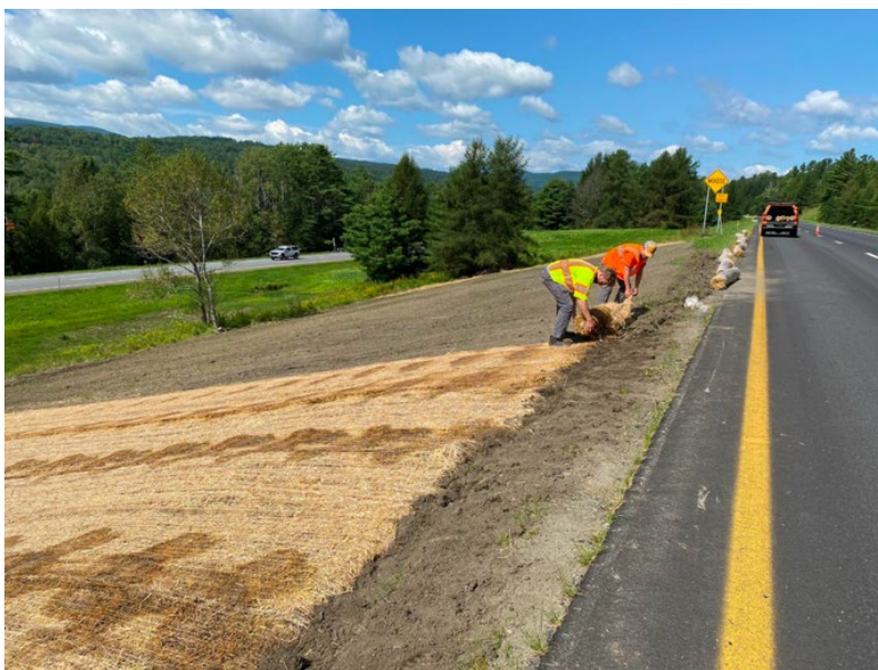
Broadcast seeding with straw matting to prevent erosion on VT's sloped site.
