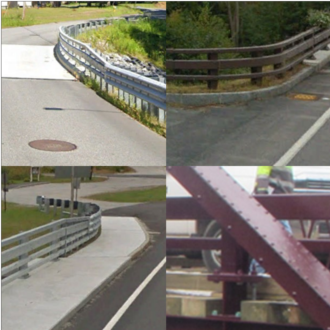
Figure 7. Examples of Atypical Installations
