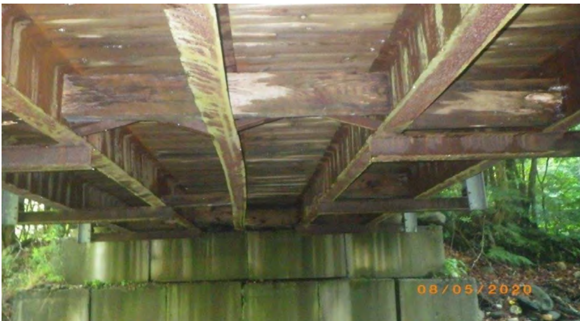
Figure 10: Example of photo of a buckled beam found in VTrans web-portal
