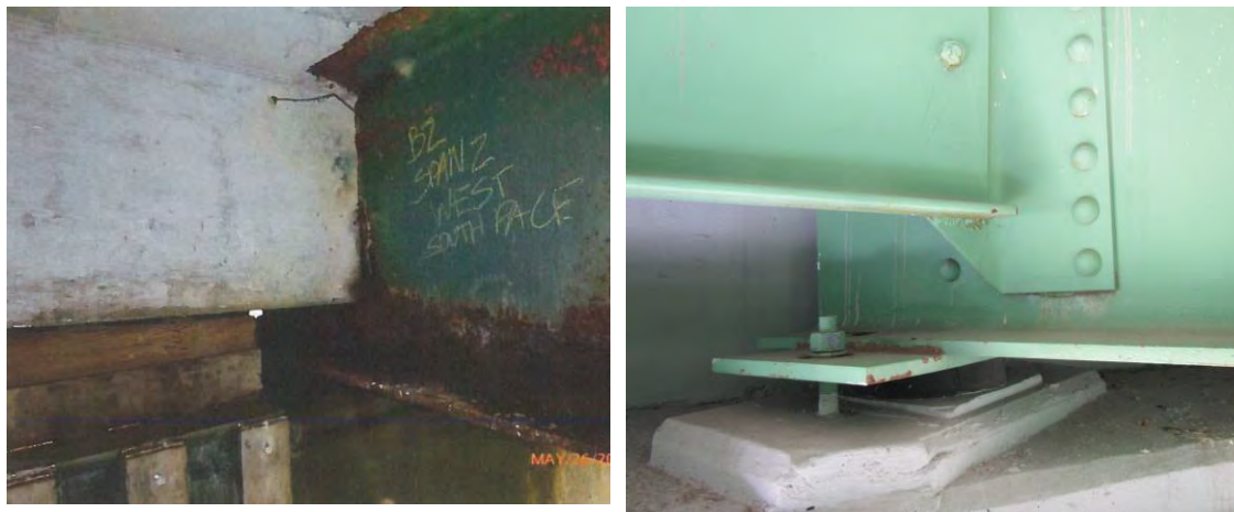
Figure 26: To the left is P-01-005 (Massachusetts) and the right structure is 042401 (Rhode Island)
