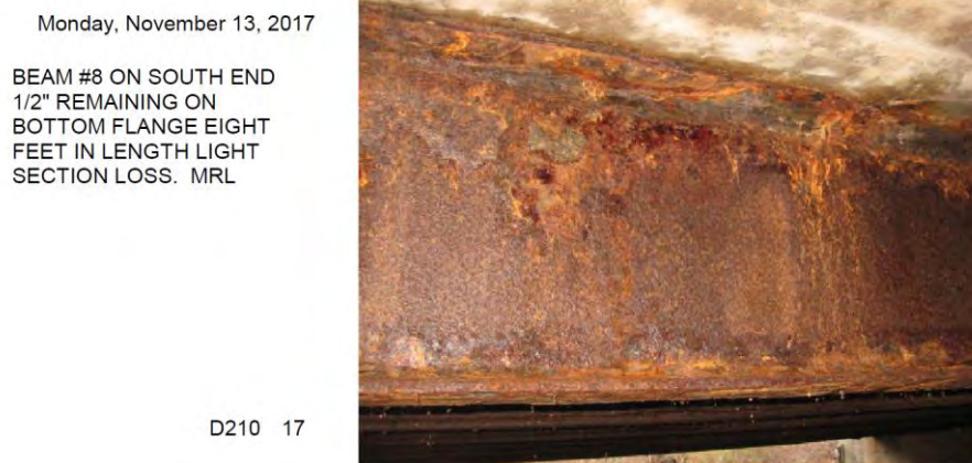
Figure 7: Example of corrosion damage taken from the records of a bridge from NHDOT
