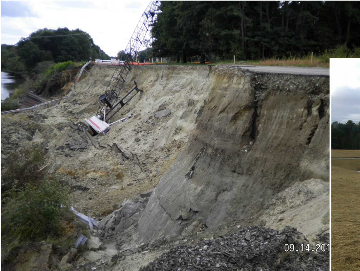
Slope Failure Summer 2010
