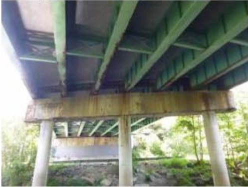
Staining unknown causation
