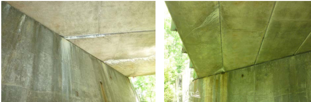
Figure 5-41: Staining of unspecified causation from gaps under beams at MA-precast_concrete_2
