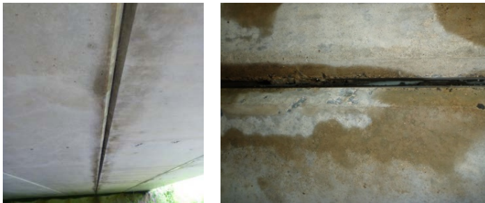
Figure 5-2: Gaps between girders in CT-concrete
