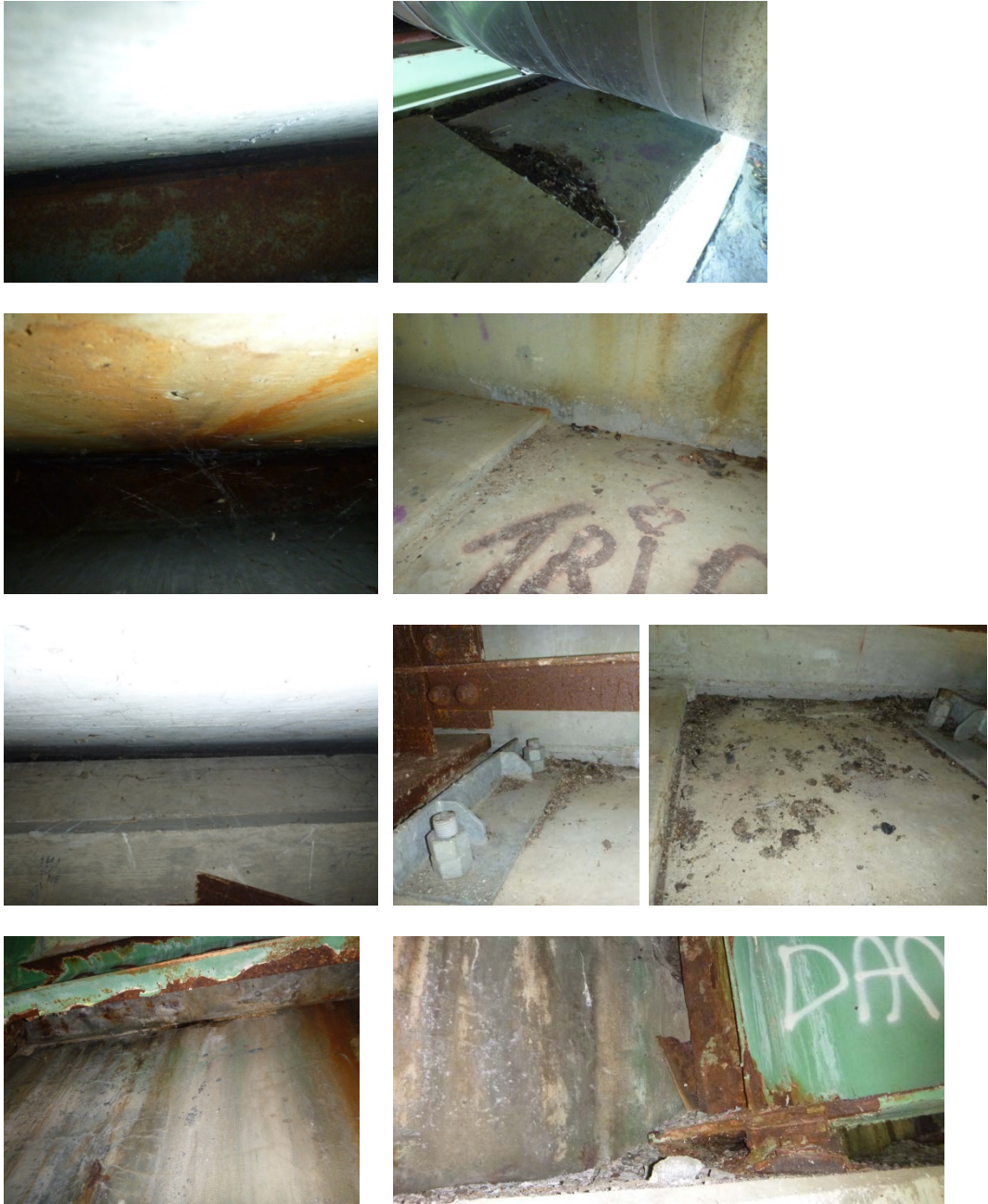
Figure 3-9: View into the expansion joint (left), and the material found below (right)
