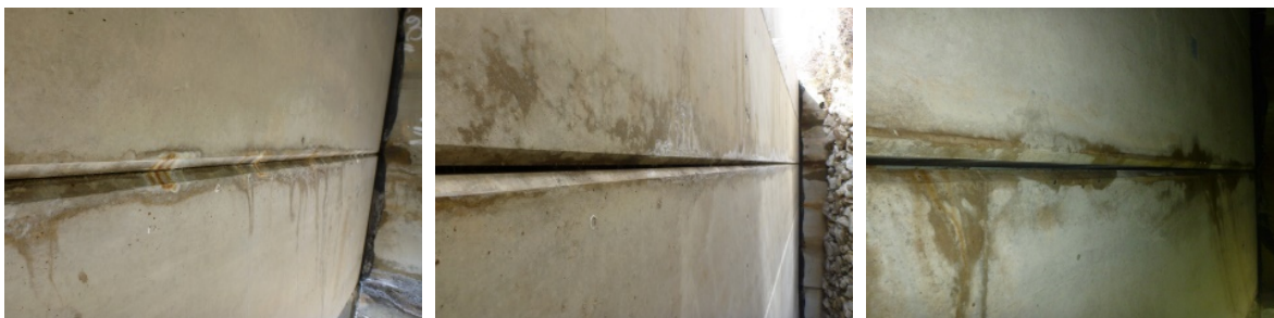
Figure 5-4: Staining of unknown causation between girders of CT-concrete
