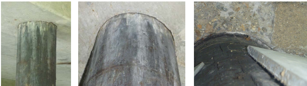
Figure 5-26: Staining on piers and gaps where piers meet deck at MA-concrete
