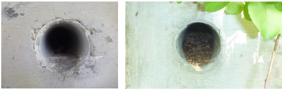
Figure 5-75: Drainage features observed in RI-concrete
