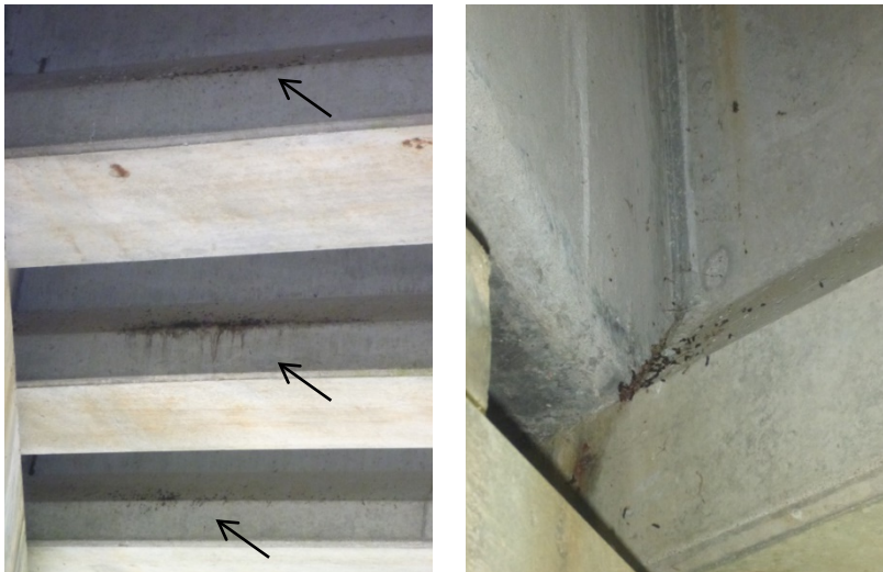
Figure 5-73: Staining evidence of roosting on bridge girders at RI-concrete
