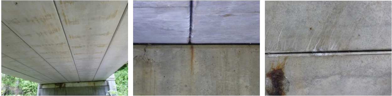
Figure 3-5: Precast concrete bridge construction leaving gaps between beams
