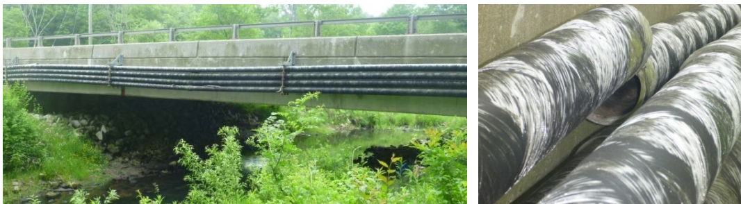
Figure 5-3: Pipes running along CT-concrete
