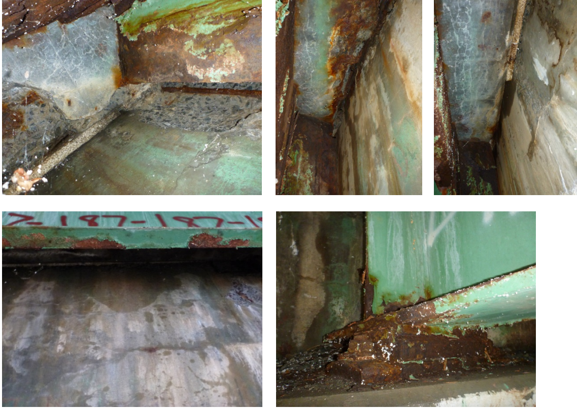
Figure 5-98: Staining caused by water damage at RI-steel_2
