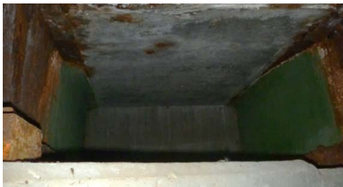
Figure 5-50: Cave-like environments near the abutments at MA-steel
