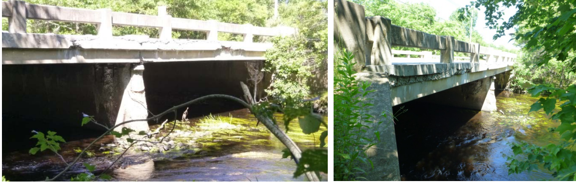
Figure 5-86: Deteriorated concrete bridge selected in RI (RI-precast_concrete_2)
