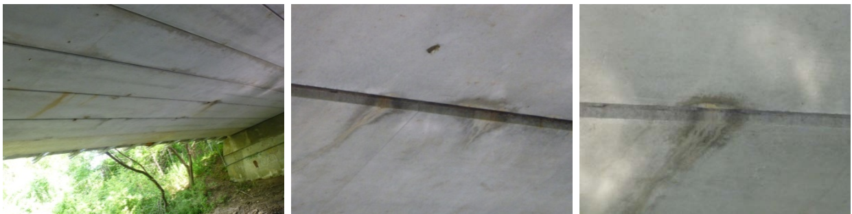
Figure 5-37: Staining in between beams in MA-precast_concrete
