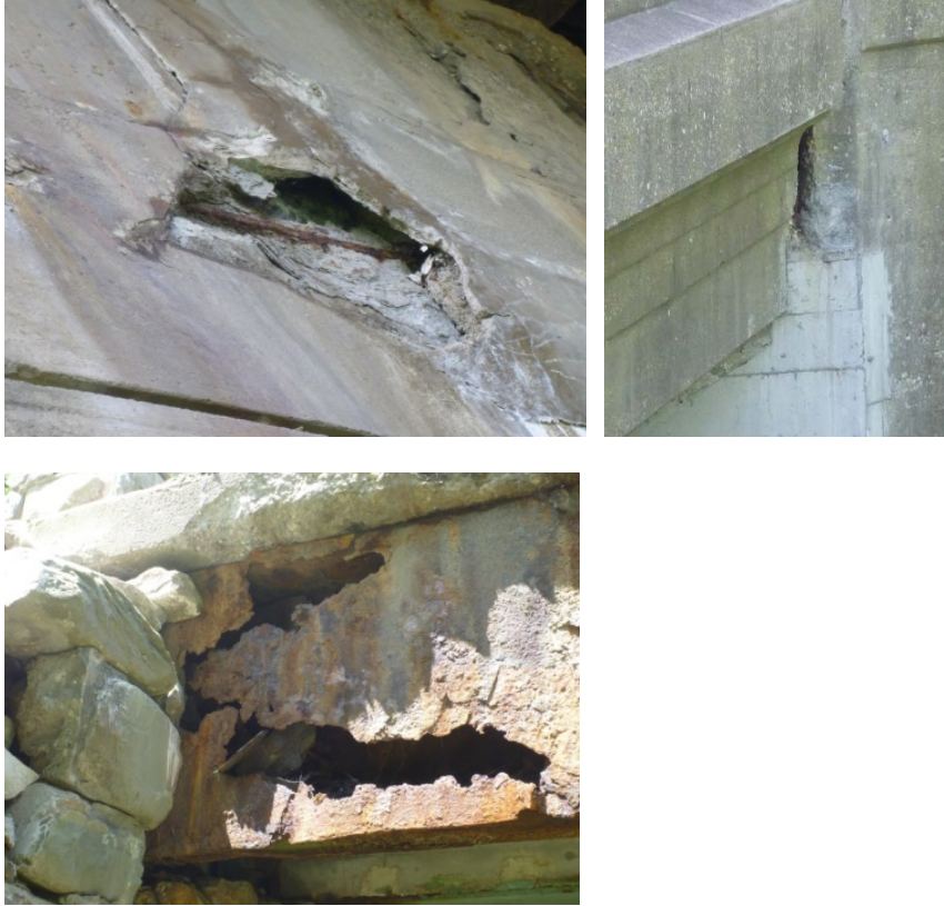
Figure 3-10: Localized deterioration creating suitable roosting crevices
