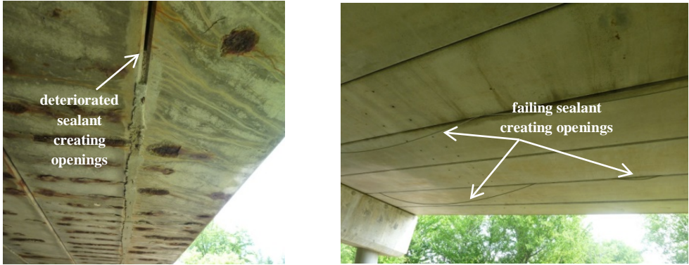
Figure 3-7: Deterioration of the sealed gaps between beams
