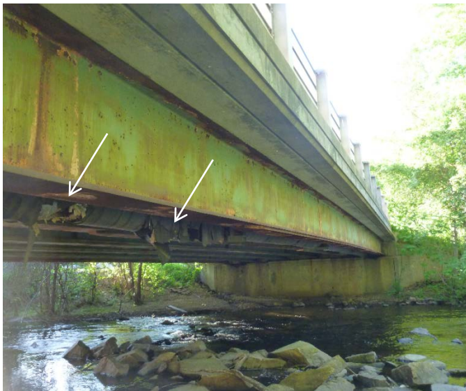
Figure 5-91: Steel construction bridge selected in RI (RI-steel) with pipe insulation deterioration (arrows)
