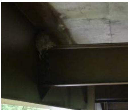
Figure 5-119: Bird's nest observed at VT-steel
