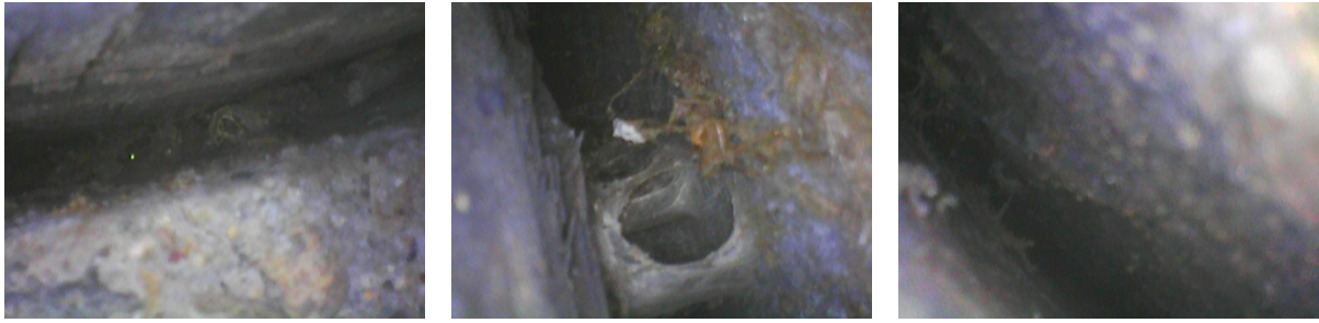
Figure 5-28: Boroscope views of crevices in MA-concrete
