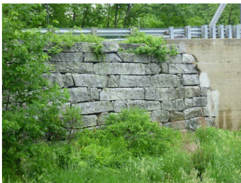
Figure 5-66: Non-grouted stone wingwalls at NH-steel_truss
