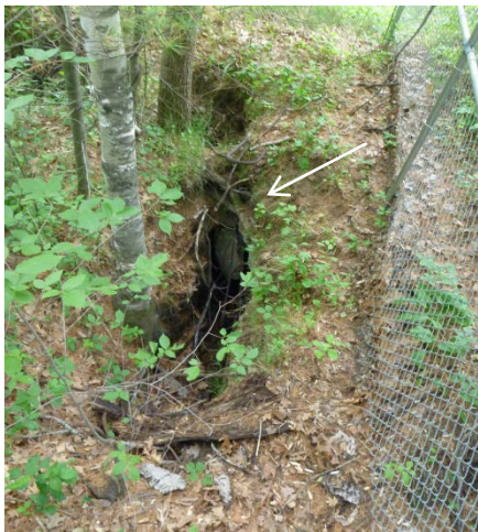
Figure 5-68: Abandoned concrete underground structure near the abutment in NH-steel_truss providing a cave-like environment and potential roost locations
