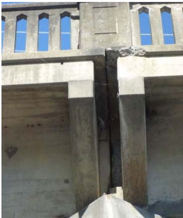
Figure 5-18: Potential roost location in the expansion joint of ME-concrete, not verified
