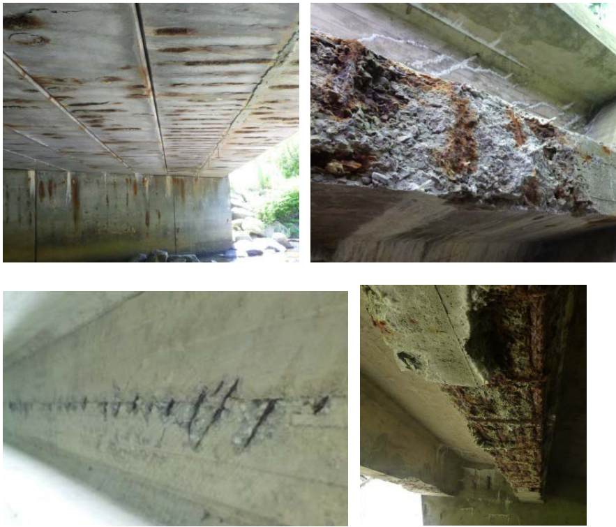
Figure 3-11: Not all deterioration will create crevices
