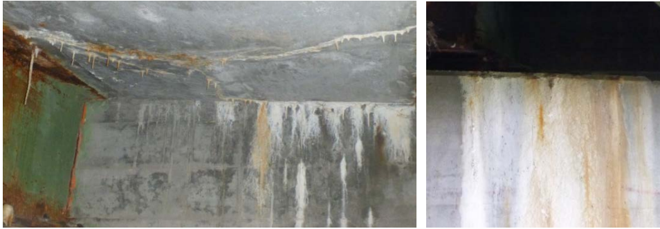
Figure 5-48: Staining of unconfirmed causation (likely structural) at MA-steel
