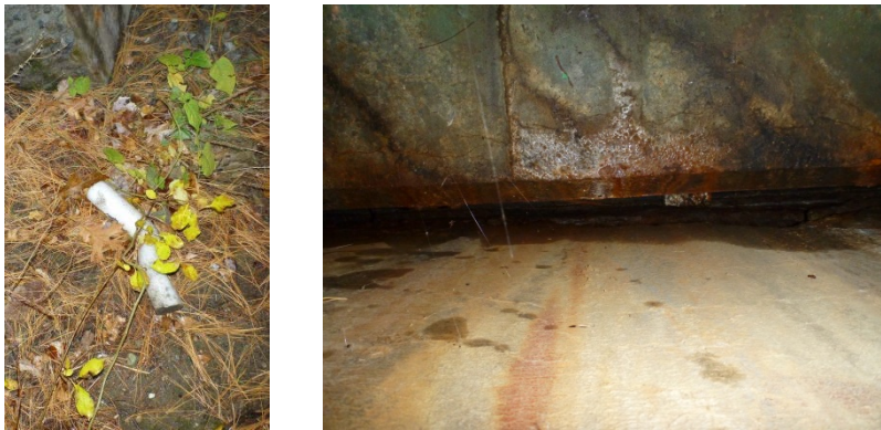
Figure 5-99: Insulation (left) that has fallen out of an expansion joint (right) at RI-steel_2
