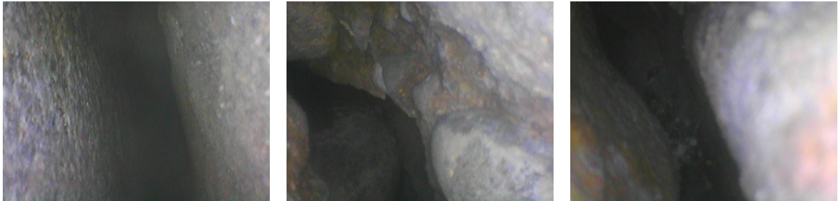
Figure 5-12: Boroscope view of gaps in non-grouted and deteriorated retaining walls by ME-concrete
