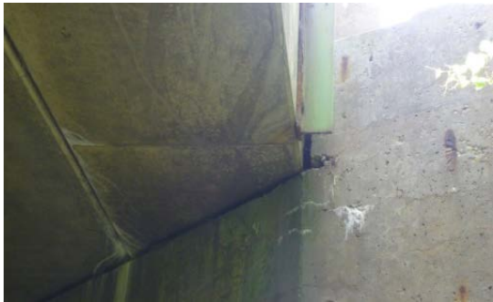
Figure 5-40: Gaps under beams at MA-precast_concrete_2
