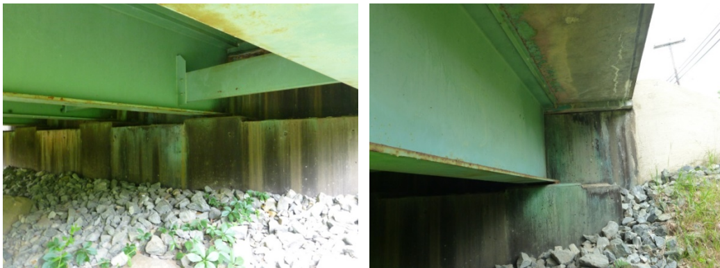
Figure 5-63: Staining observed at the abutments in NH-steel (likely structural)
