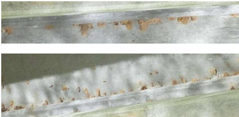
Figure 5-76: Mud-Dauber's nests observed on girders of RI-concrete
