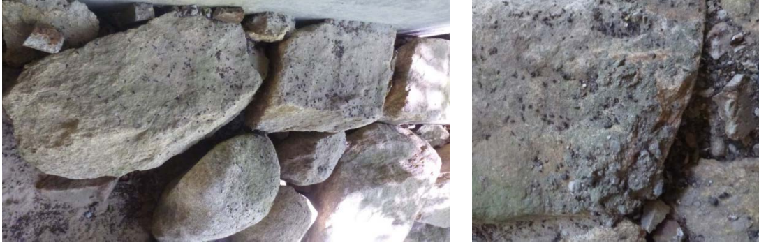
Figure 5-74: Guano evidence of roosting at RI-concrete (confirmed EPFU)
