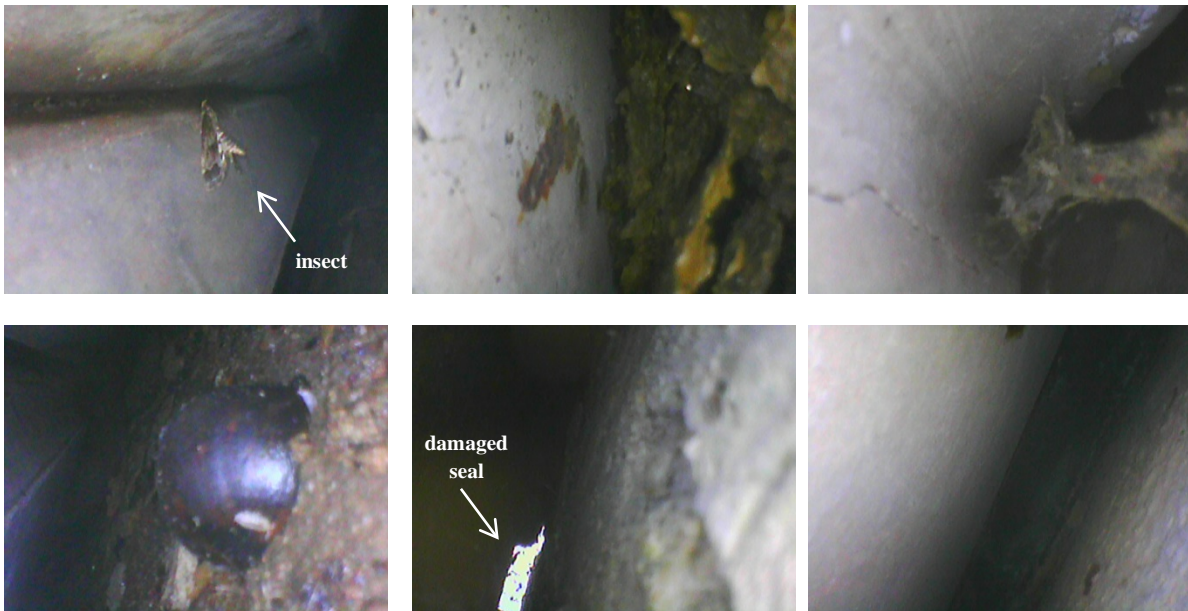
Figure 5-83: Boroscope view between girders and between girders and the abutment at RI-precast_concrete showing insects, debris, structural components, sealant damage, and clean gaps
