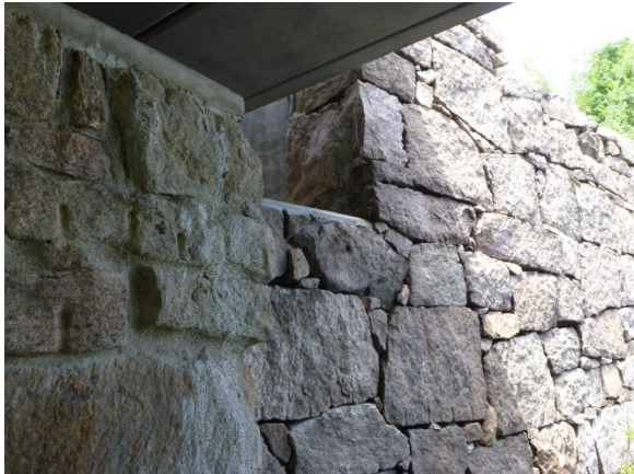
Figure 3-15: Construction with grouted stonework and non-grouted stonework (left and right sections of photo)
