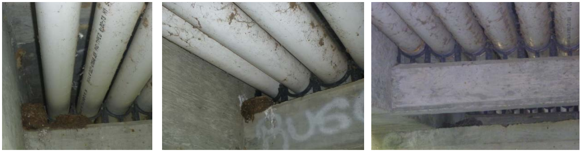
Figure 5-30: Birds' nests and pipes observed at MA-concrete
