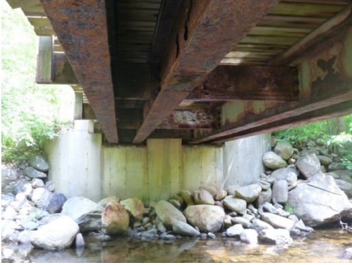
Figure 5-20: Significant deterioration and staining in ME-steel/wood
