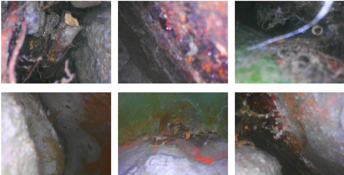
Figure 5-53: Boroscope views into cracks showing debris in crevices at MA-steel
