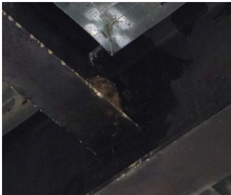
Figure 5-69: Bird's nest at NH-steel_truss
