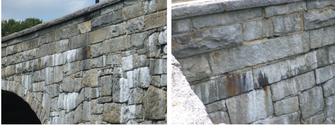
Figure 5-58: Roosting crevices and staining on the stone façade in NH-concrete_arch
