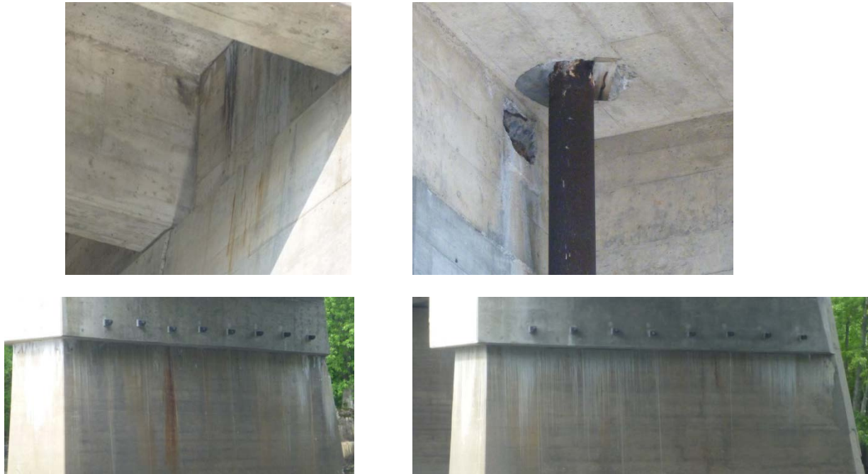
Figure 5-14: Staining of unknown causation at ME-concrete
