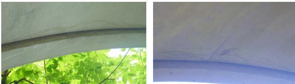
Figure 5-107: Staining of unspecified causation by gaps in VT-concrete_arch
