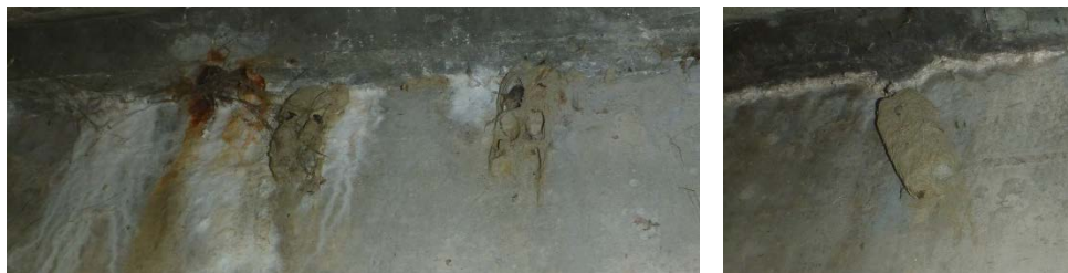
Figure 5-6: Mud-Dauber's nests observed on CT-concrete
