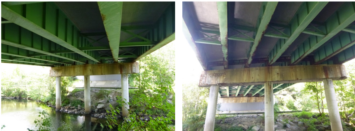
Figure 5-101: Staining of unidentified causation in the center pier of RI-steel_2
