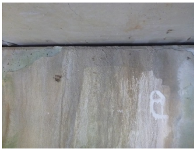
Figure 5-82: Staining of unidentified causation between the girders and where the girders and abutment meet in RI-precast_concrete
