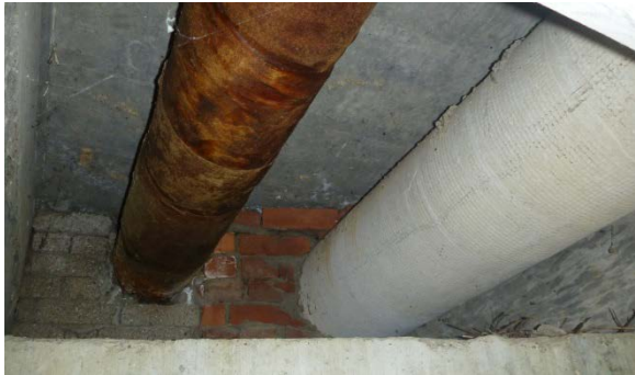
Figure 5-29: Pipes observed at MA-concrete
