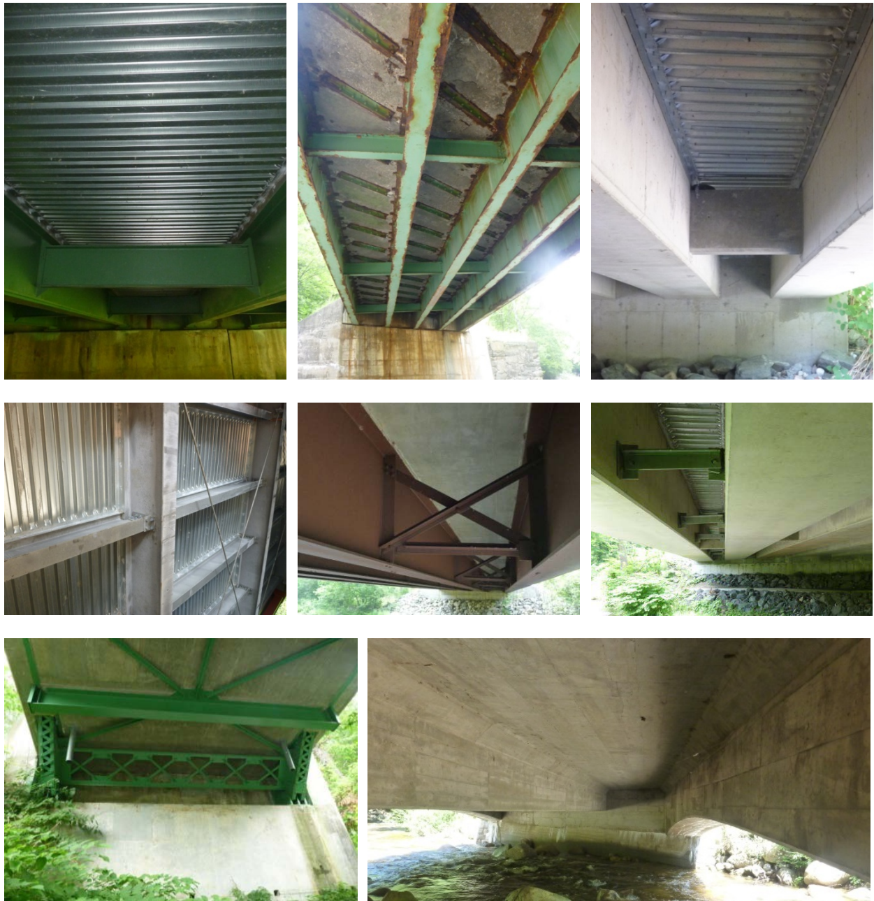
Figure 3-18: Bridge deck construction that does not create suitable roosting crevices and locations
