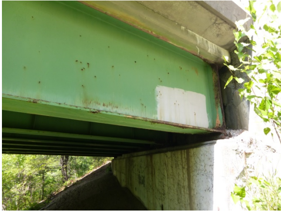
Figure 5-95: Abutment under which the dead bat was found at RI-steel_2
