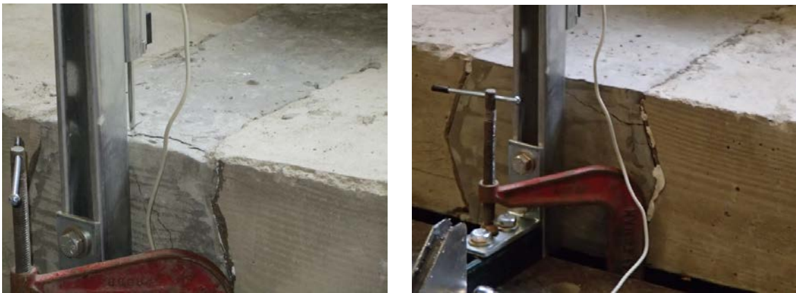
Figure 6-10: Crack in the Joint: Specimen 1 (left); Specimen 2 (right)
