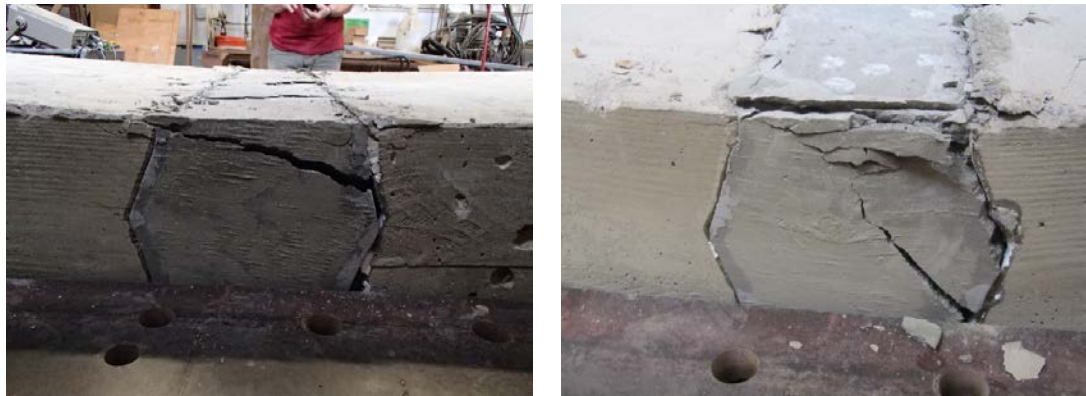
Figure 6-16: Detail View (Back) of the Joint after Failure: Specimen 1 (left); Specimen 2 (right)
