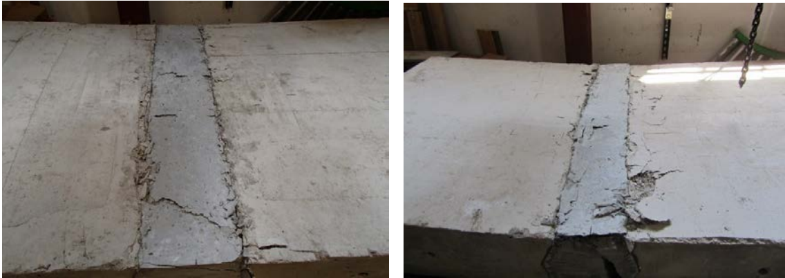
Figure 6-14: Top View after Failure: Specimen 1 (left); Specimen 2 (right)
